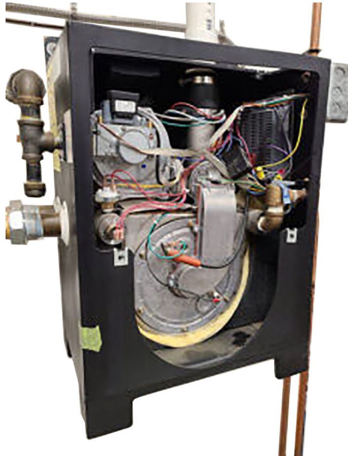
Figure 28 Wall-mounted Mod/Con Boiler. (Rod Lidstone) CC BY 4.0 ( https://creativecommons.org/licenses/by/4.0/legalcode.en )
