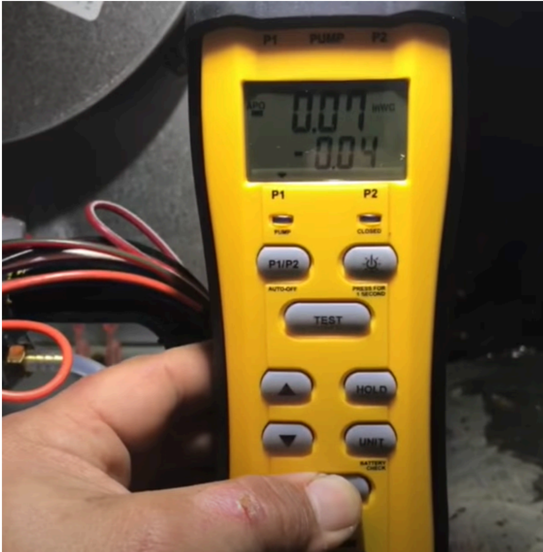
Using a Manometer for Gas Pressure (Rheem Furnace) (HVAC tips ( https://www.youtube.com/watch?v=pE03Zt8zVxg ), 2020 (video still: 4:18). Used under Fair Dealing for educational purposes.
