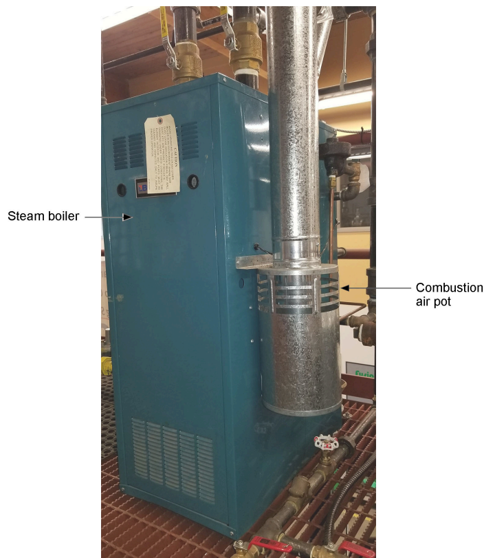
Figure 2 Combustion air pot on a steam boiler. (Skilled Trades BC, 2021) Used with permission.
