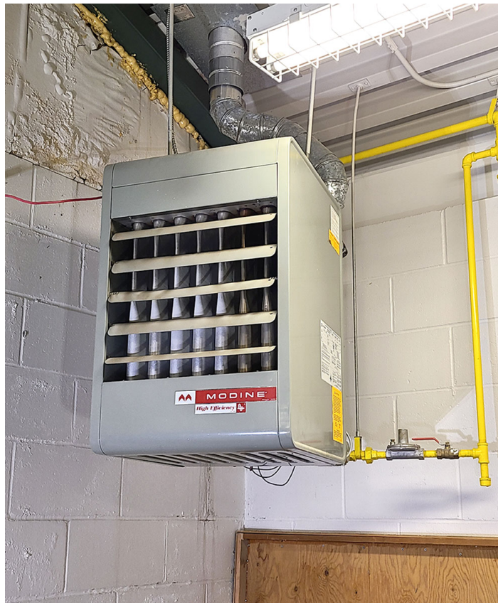
Figure 8 Suspend gas fired unit heater. (Rod Lidstone) CC BY 4.0 ( https://creativecommons.org/licenses/by/4.0/legalcode.en )
