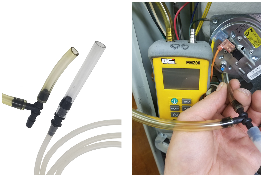
Figure 18 Barbed reducer and barbed tee (left), manometer being connected into pressure switch sensing line (right). (Rod Lidstone) CC BY ( https://creativecommons.org/licenses/by/4.0/ )
