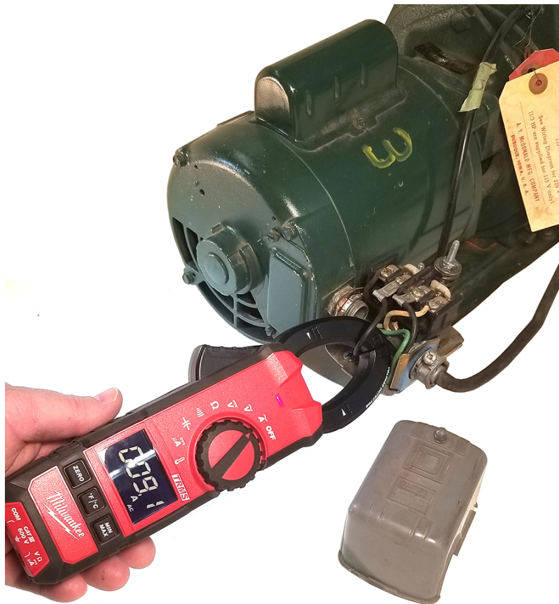
Figure 10 Using the clamp meter to measure pump motor amperage. (Skilled Trades BC, 2021) Used with permission.
